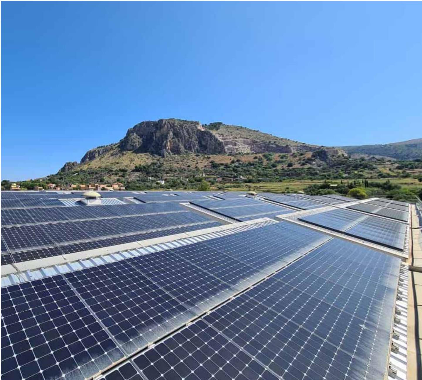
Aspra photovoltaic plant Plant power: 336 kW Plant size: 1100 panels
